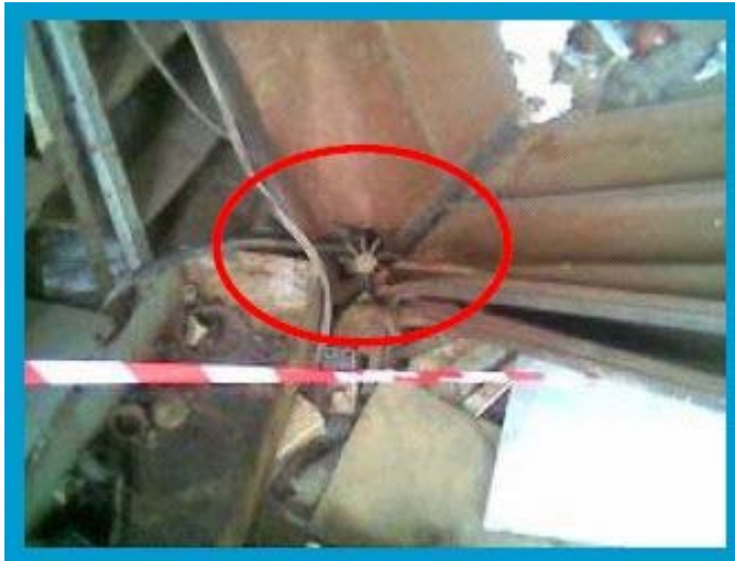
Unexploded mortar found inside a building in Abyei
