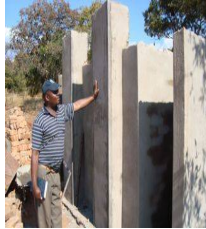
IMC is constructing latrines at Health centres as part of an ECHO-funded project to strengthen preparedness at community and facility level
