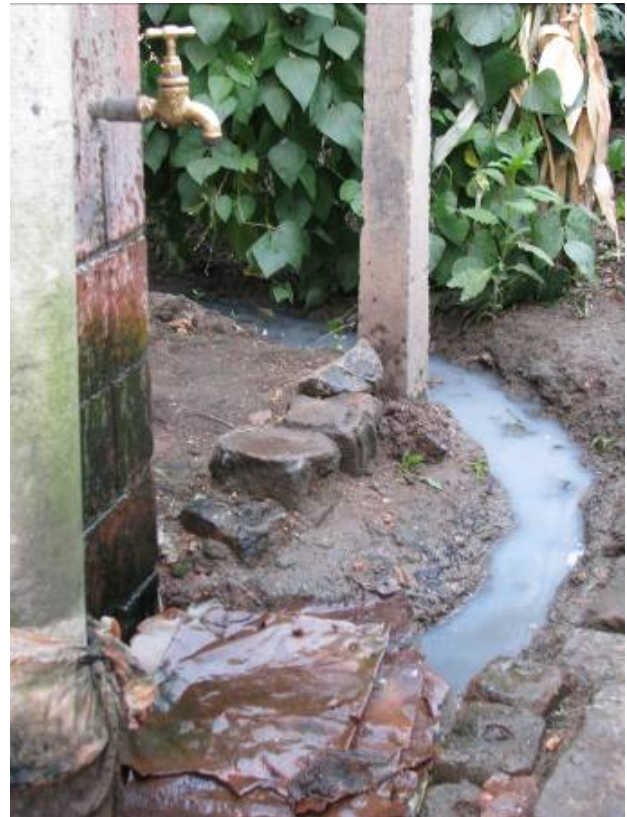
This home in Makokoba, Bulawayo, reflects the urgent need for support towards rehabilitating WASH facilities. Photo courtesy of Richard Johnson. OCHA-VMU.
